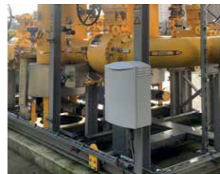
The correlative measuring device gasQS flonic in the control cabinet at the gas transfer station
